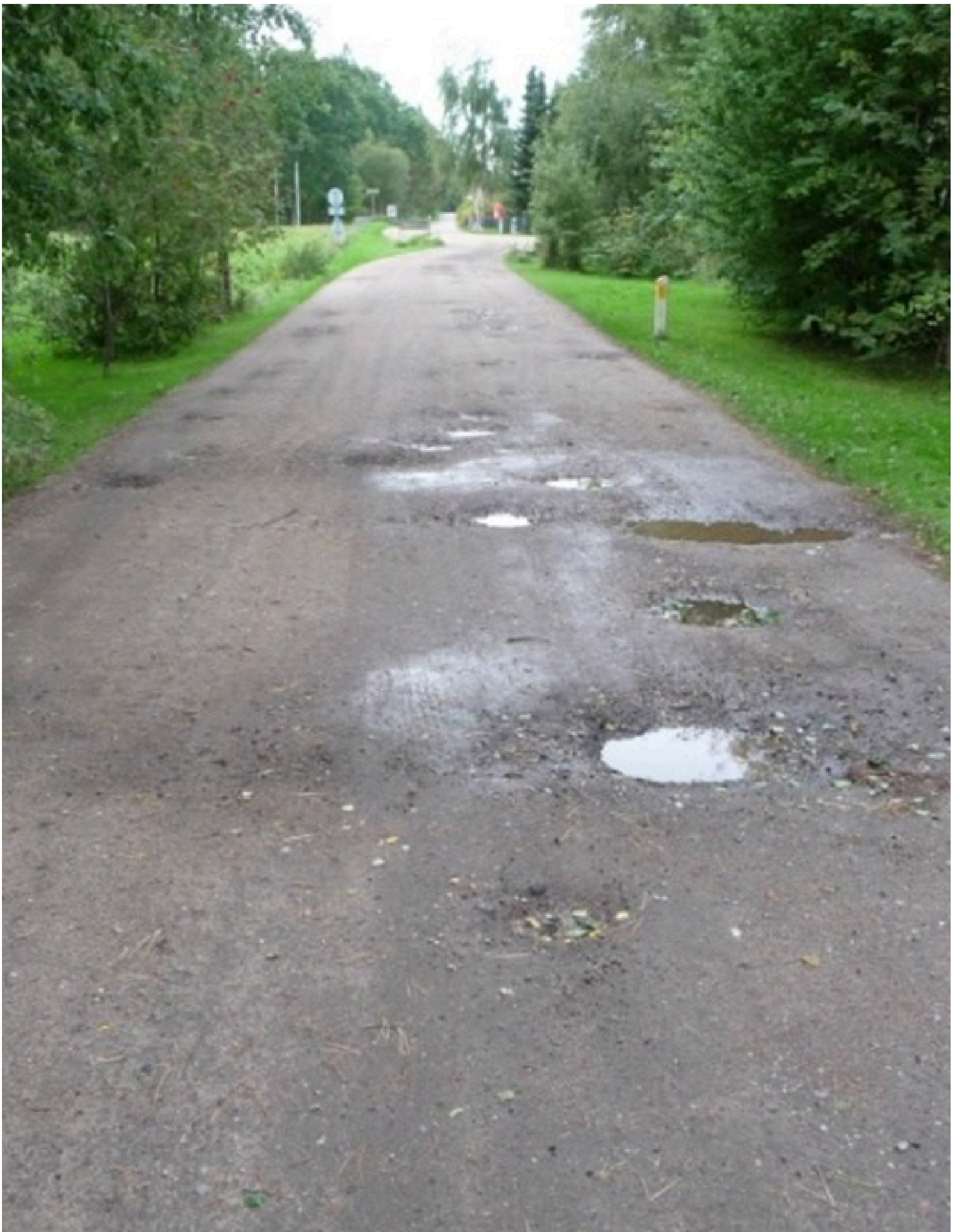
Gravel road with potholes.
