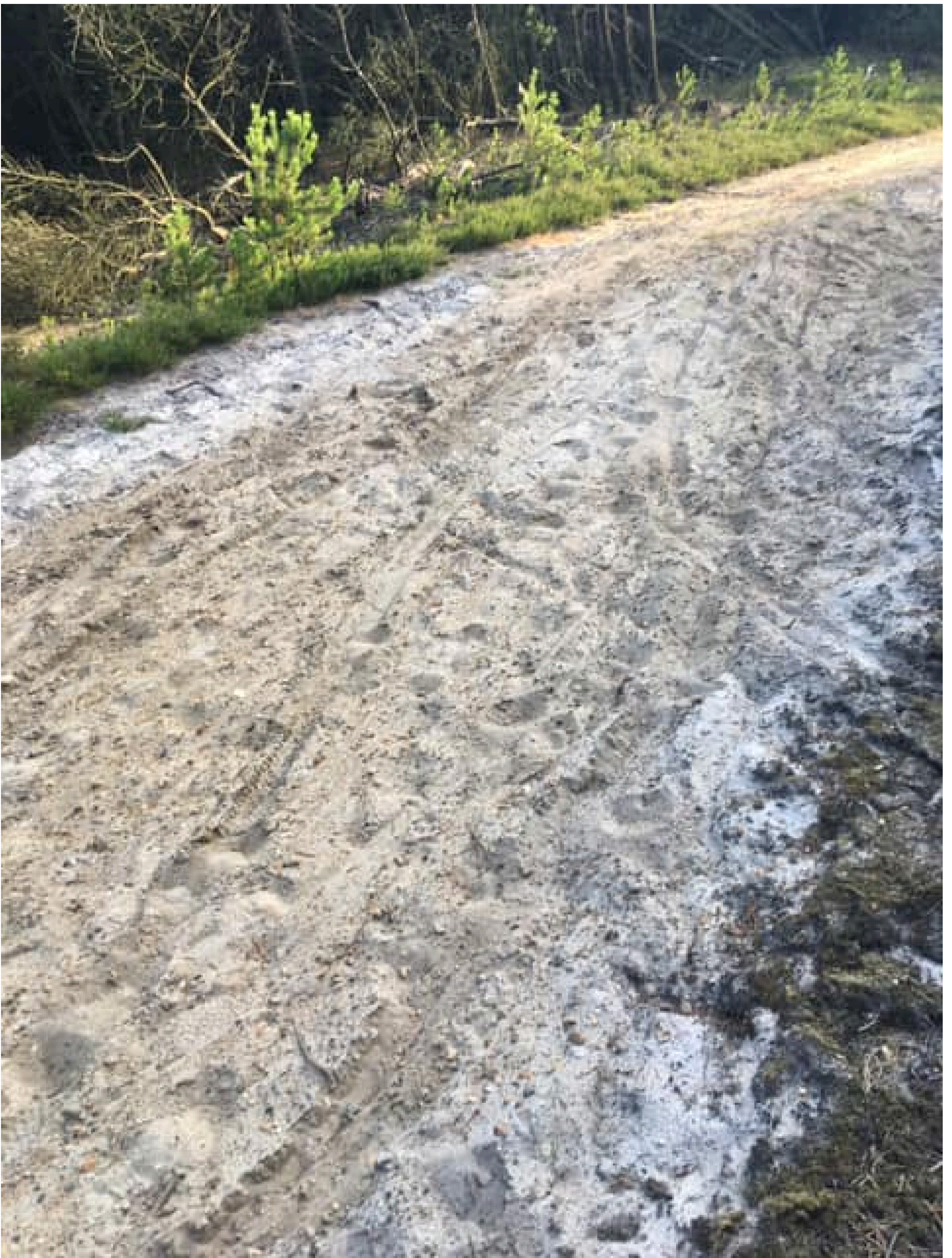
Loose and sandy due to hot weather.
